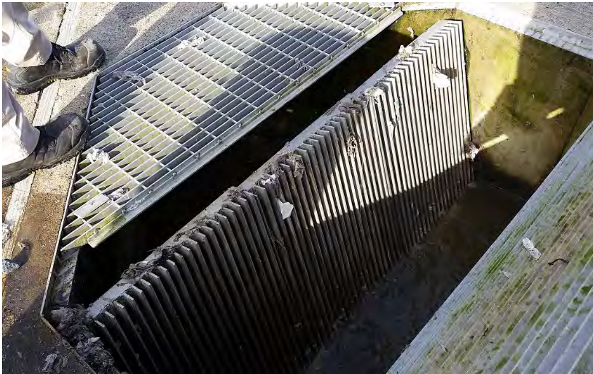
FIGURE 3-4: EXISTING BAR SCREEN
